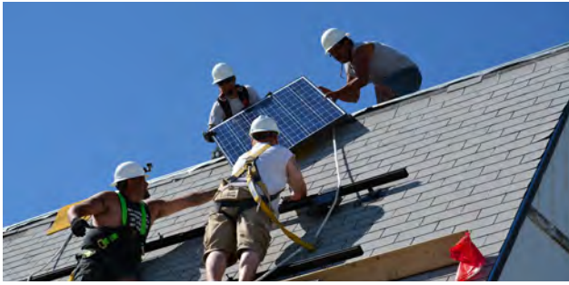
Henry Red Cloud (top right) and his crew of Lakota Solar Enterprises workers install solar panels at KILI Radio, Pine Ridge, South Dakota. Photo by Lisa Olken.
